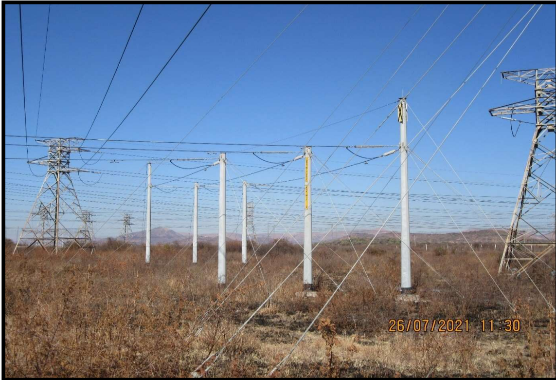
Figure 9: Existing low-lying D-DT 7618 tower structures taking power from Ararat MTS which are proposed for Ararat Alternative Route A
