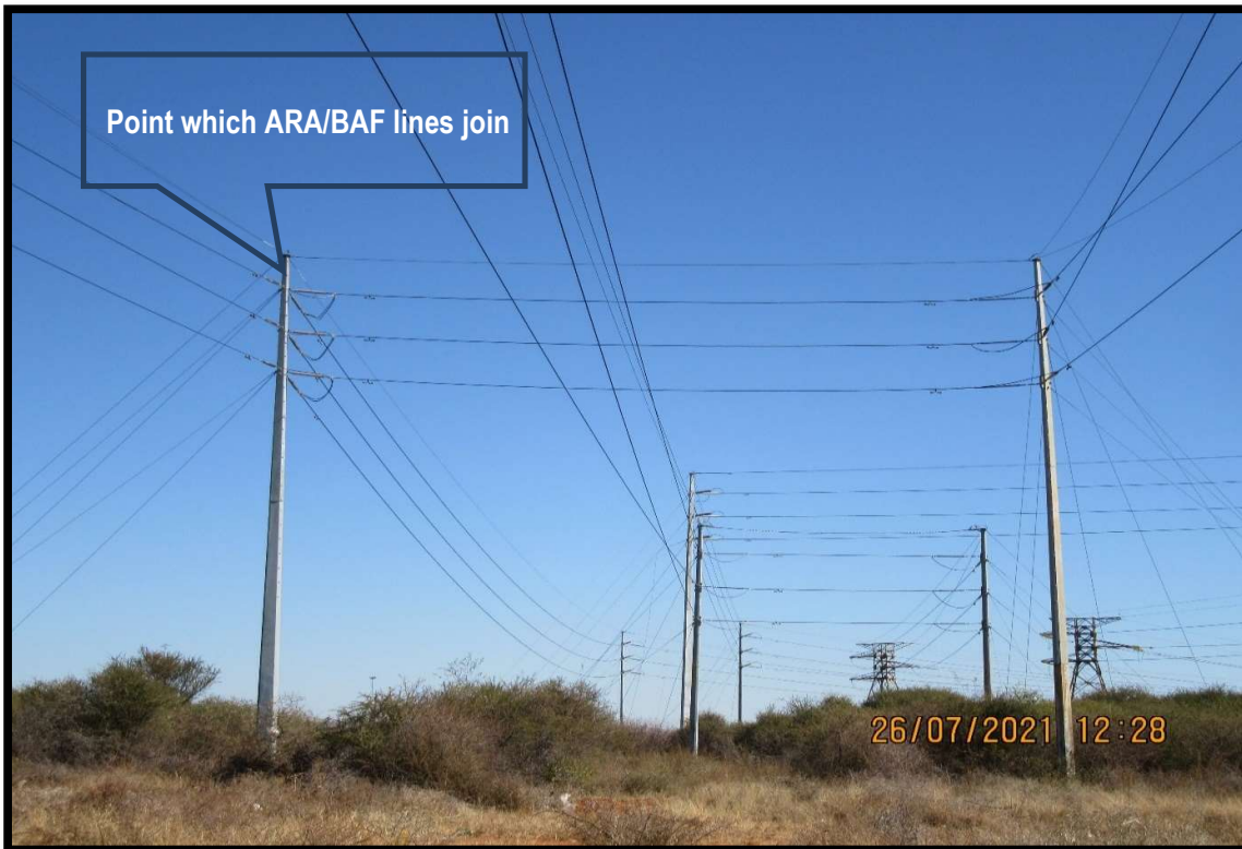
Figure 12: Image showing point at which the ARA/BAF lines from Ararat MTS join into one single line into Bafokeng 7 substation
