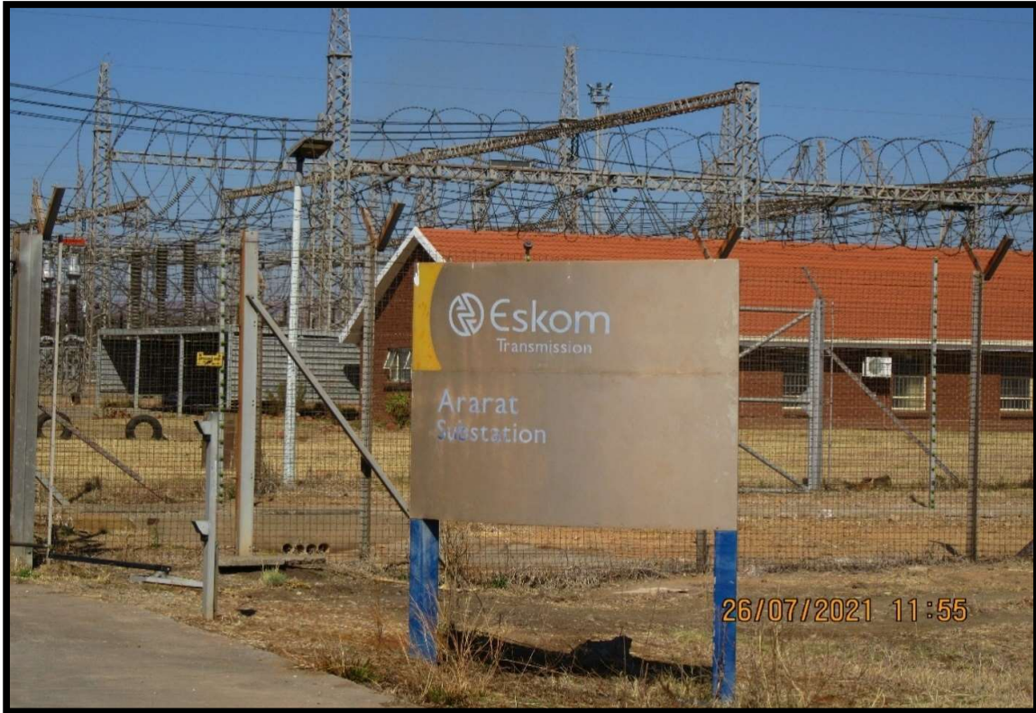
Figure 7: Entrance to Ararat Main Transmission Substation
